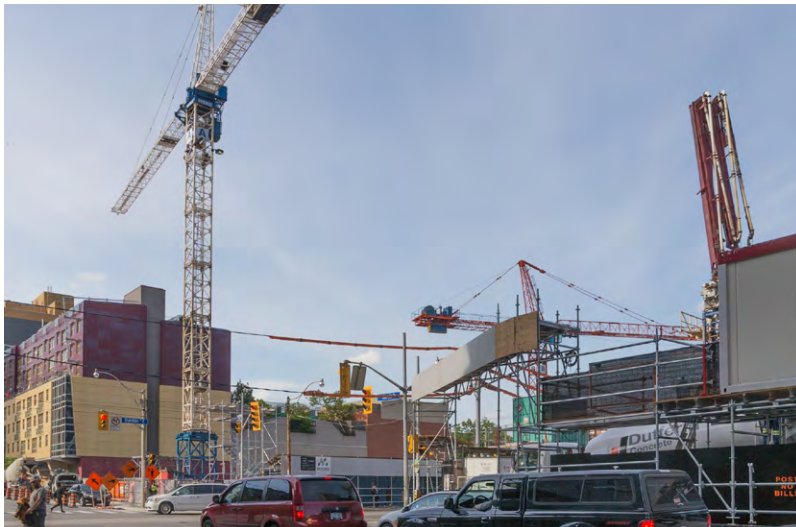
Construction cranes at the corner of Dundas Street East and Jarvis Street (Photo by Dominic Ali)
